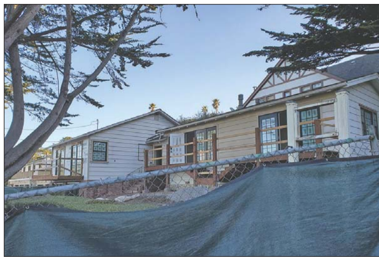
Construction is underway at the former Colonial Terrace, which is being rebranded as the Carmel Beach Hotel and is set to open in the spring and will include a guest-only restaurant run by chef Justin Cogley.
