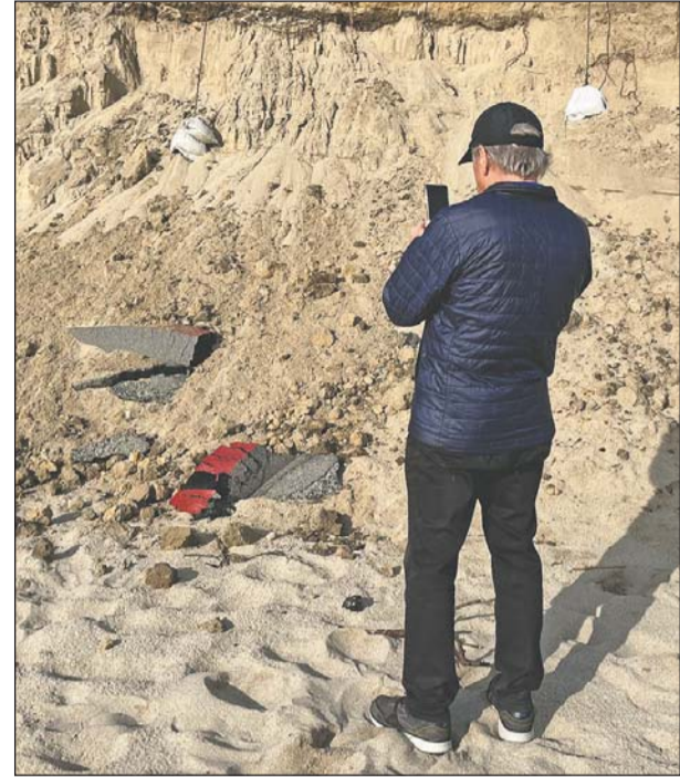
Resident Lorin Letendre photographs chunks of asphalt that have broken off of Scenic Road and tumbled down to the beach below.
