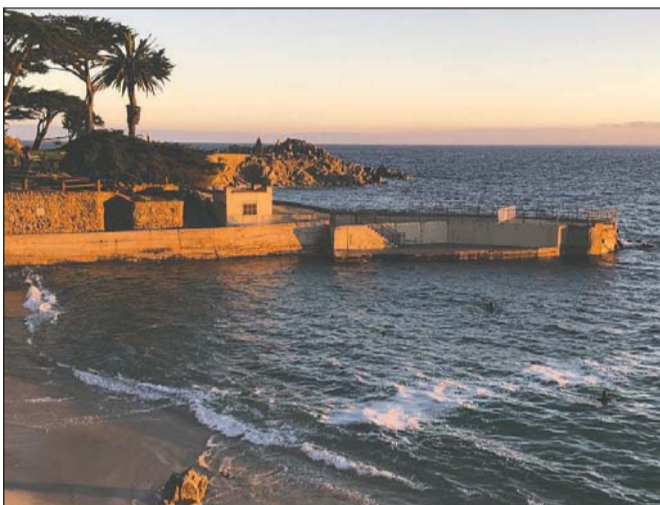
The Pacific Grove City Council earlier this month OK'd a plan for an engineering firm to assess the Lovers Point Pier, the tip of which was heavily damaged in a storm. The city may opt to fix the structure.
