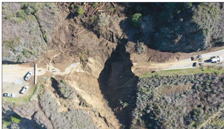
One of Big Sur's lesser known coastal tributaries, Rat Creek is in the news because the bridge over it collapsed during recent storms. Caltrans is still assessing how it will fix the highway, and how long it will take.
