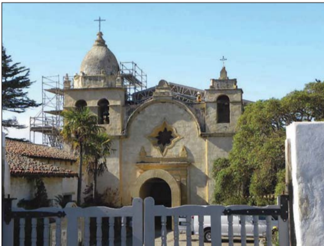
During the first phase of renovation at Carmel Mission in 2012, workers removed the roof from the Basilica so they could drill into the adobe walls and reinforce them with steel rods. The same is set to be done to the Sir Harry Downie Museum.
