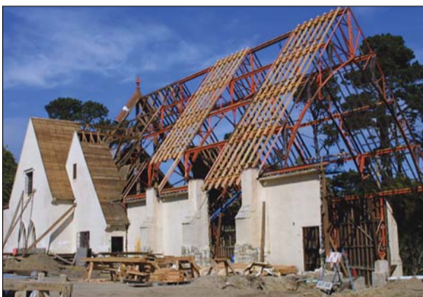
Sunset Center undergoing reconstruction in 2002. The bonds used to pay for its renovation have been refinanced — again.
