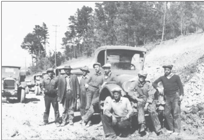
Workman in 1929-30 building a new road – now known as the Holman Highway – to shorten the distance between Carmel and Pacific Grove.
