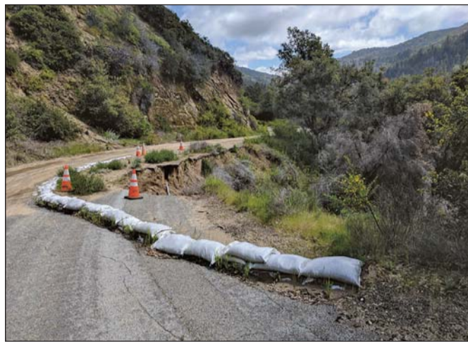
Three years after winter rains triggered mudslides that badly damaged Palo Colorado Road, the upper portion of the narrow and winding route is still closed. But last month, the county allocated $500,000 to jumpstart the design and planning process for the work.
