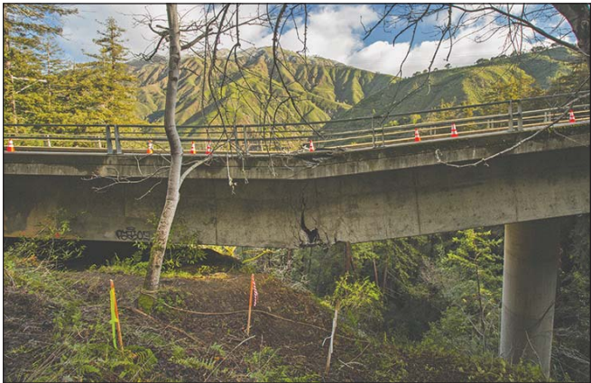
In 2017, Pfeiffer Creek Bridge in Big Sur failed (left), and Highway 1 was closed for 7 months while a new bridge was built. Caltrans officials say there's no need to worry about the safety of Bixby Bridge (below) or other Big Sur bridges, although they concede they will all one day need to be replaced.
