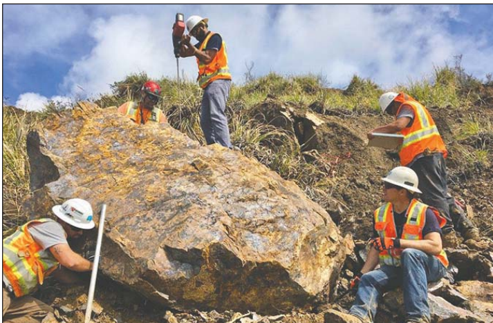
A boulder that posed a threat to motorists at Paul's Slide in Big Sur is prepared for demolition by a Caltrans crew March 8.
