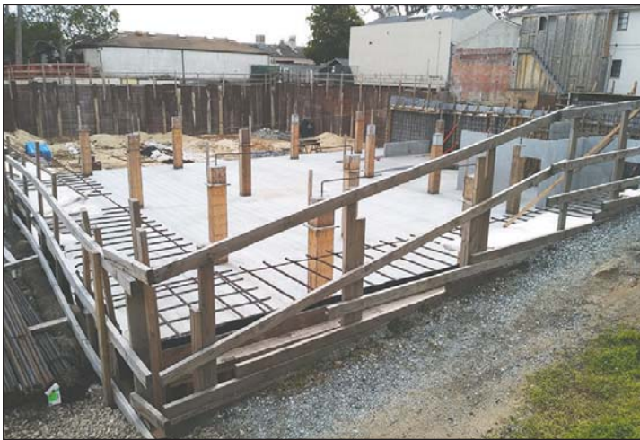
Construction of a large mixed-use complex at Dolores and Fifth has proceeded very slowly since it began in the summer of 2017, due to logistical challenges resulting from the project's doubling in size a year ago, and the need to get a new loan.
