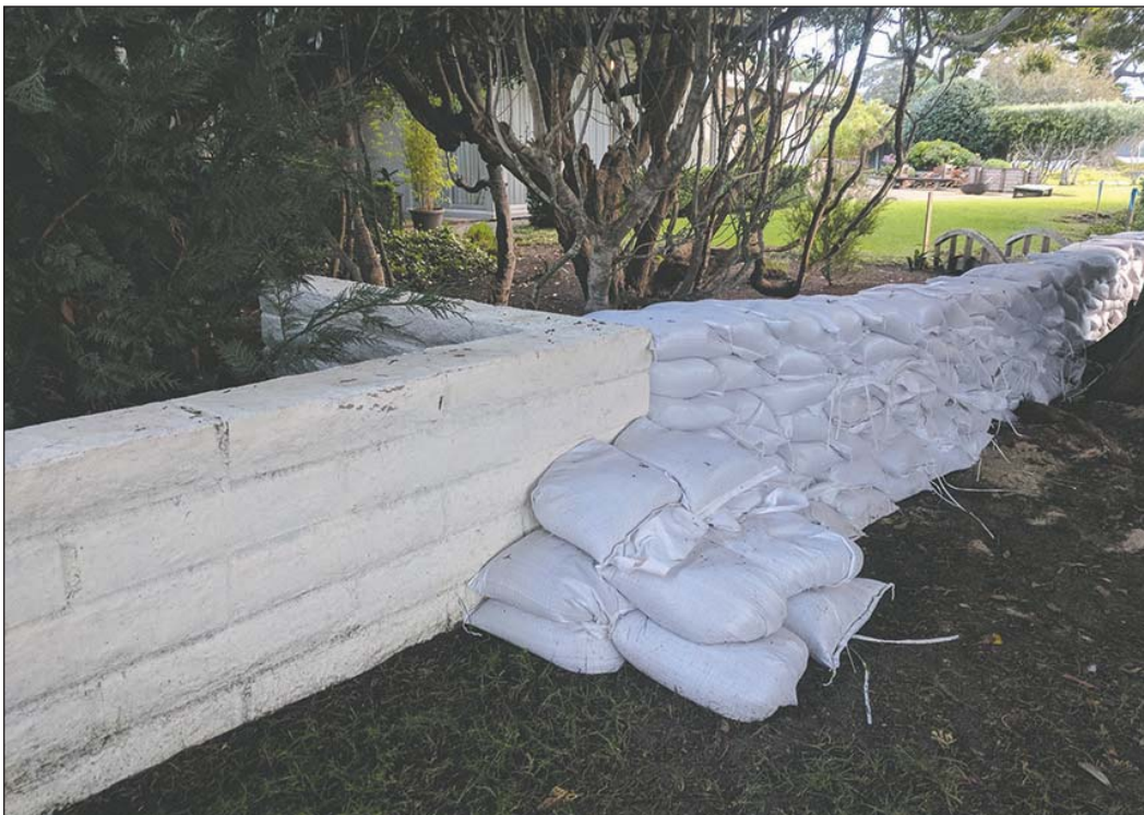
A 2-foot-high wall installed by a homeowner to reduce the risk of flooding meets a stack of sandbags that county workers installed next to his neighbor's home.
