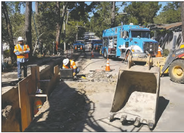
PG&E crews worked to stop the flow of gas at Carpenter and Fifth Monday after a city-hired contractor hit a high-pressure main with a backhoe. They then used sniffers to ensure no gas lingered in water and sewer lines in the area.
