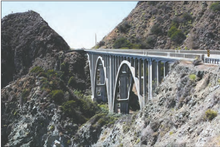
To remove corrosion due to salt contamination from Big Sur's Big Creek Bridge, a $21 million project will begin sometime next year. The work will be paid for with taxpayers funds from SB 1.
