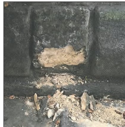
Crumbling stones will finally be replaced in the World War I memorial arch, thanks to volunteers who worked to find the stone and are raising money. A year ago, city officials and others met at the arch to discuss the options.
