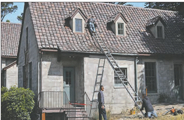
Roofers used custom-made tiles to repair leaks at the city's historic Flanders Mansion Thursday. The city council will be discussing its fate again sometime in the coming months.
