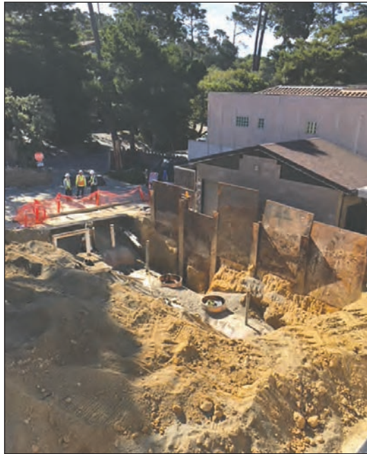
Crews used heavy equipment to break up the concrete slab and dig a giant pit to remove the public works fueling station.
