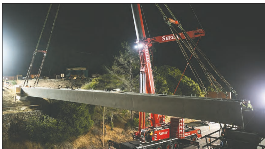
Construction crews Tuesday night installed these tub girders over Highway 68 in Monterey for a pipeline that will deliver drinking water to the Monterey Peninsula.
