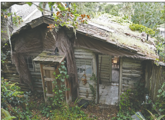
This 112-year-old cabin on Monte Verde Street is so riddled with termites, beetles and dry rot that it's falling apart, but the historic resources board isn't ready to let the owners tear it down.
