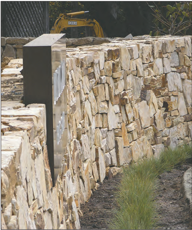
Residents have complained about this new rock wall at the entrance of Ventana Inn, and they are wondering why it wasn't reviewed by the Big Sur Land Use Advisory Committee.
