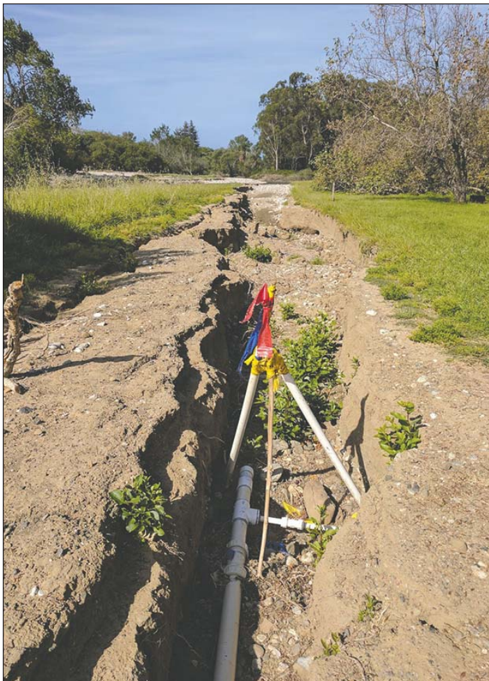
This trail at Andrew Molera State Park is still closed due to storm damage, but another route that provides access to the park's popular beach is now open, and other trails are expected to open soon.
