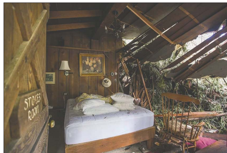
The cabins at Deetjen's suffered major damage from falling trees during winter storms. Deetjen's chef will be doing a pop-up dinner at the Big Sur Roadhouse Friday night to raise money for the beleaguered property and its employees.
