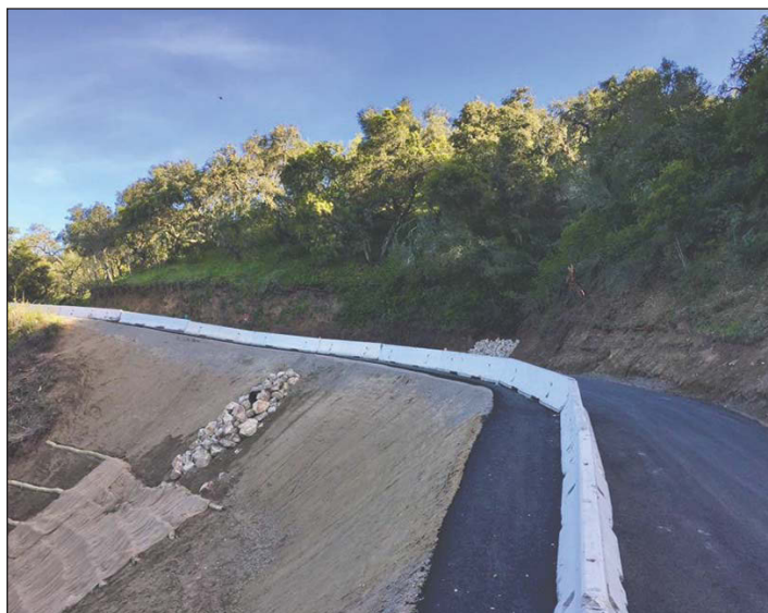
Asphalt and k-rail were the last elements necessary before a temporary single lane could be opened on Cachagua Road. The road opened April 1, giving residents much to cheer about.
