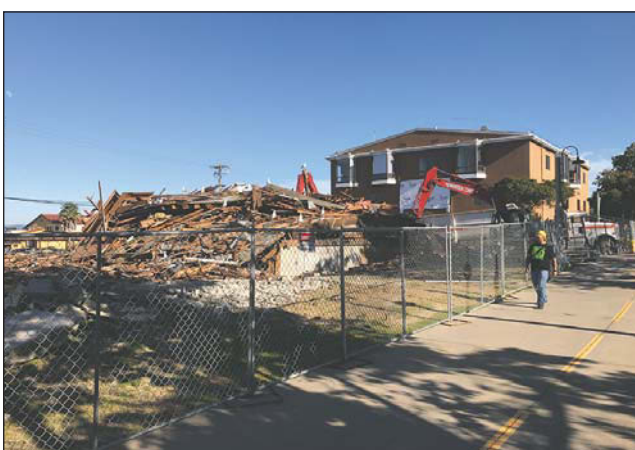
On Wednesday, the Monterey Bay Aquarium completed demolition of a former retail building at 625 Cannery Row to make way for a $50 million, 13,000-square-foot student education center. Aquarium spokesman Hank Armstrong said extra caution was taken to demolish the structure so the building next door was not damaged. Construction of the new center is expected to begin soon.
