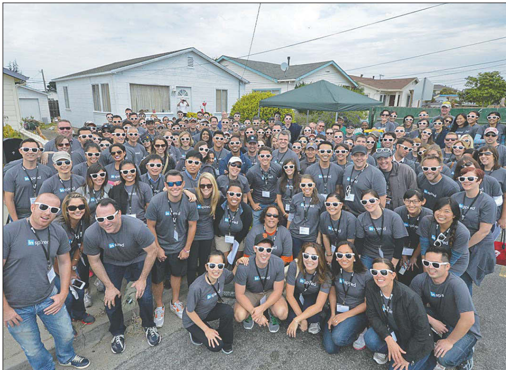
Obviously the cool kids, this group of locals and LinkedIn employees rehabilitated three homes on one block in Seaside in 2013 as part of Rebuilding Together: Monterey/Salinas.
