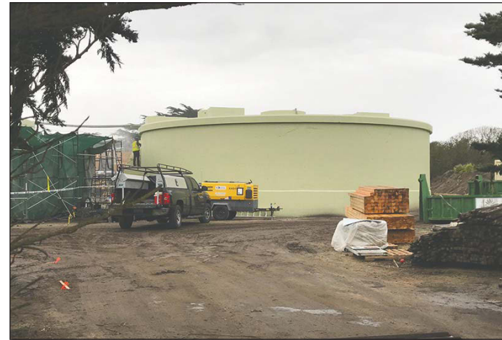
A worker on Thursday power washed this large tank, which is part of Pacific Grove's old sewer plant that will be used for a new water recycling project.
