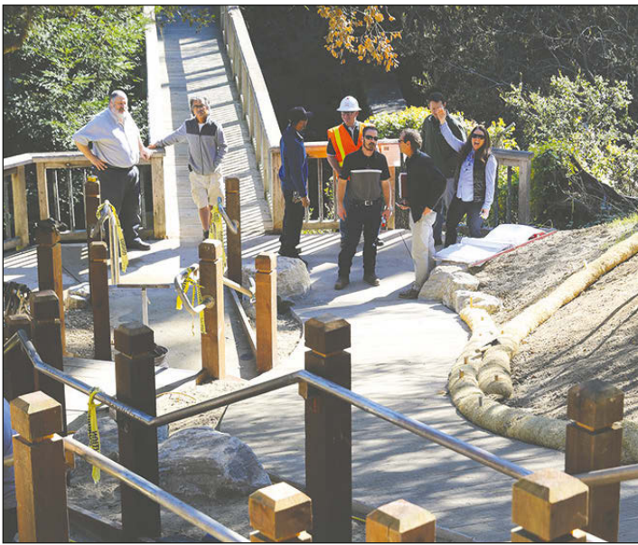
Public officials checked out the new entrance to Mission Trail park Thursday morning. Access at Mountain View has been closed for construction of the new stairs, ramp and other improvements since early August.
