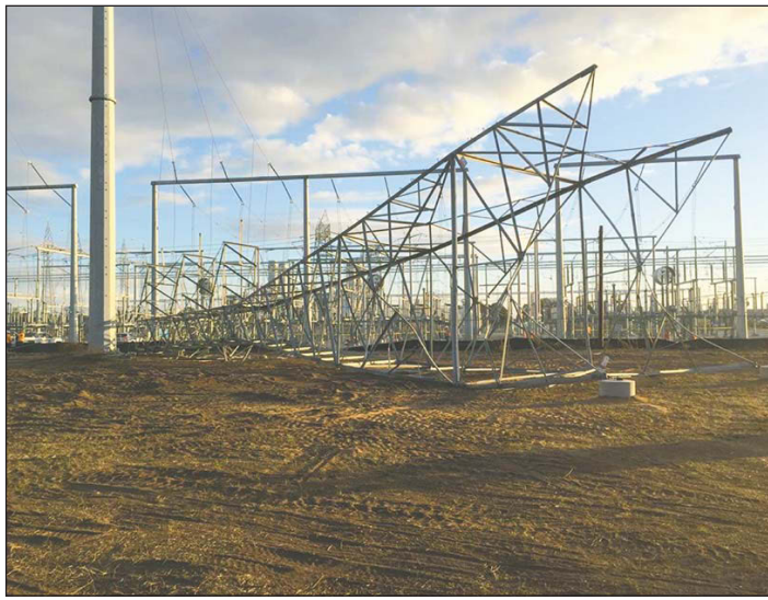
This PG&E transmission tower at the Moss Landing power plant fell over during calm weather last fall, leaving more than 50,000 people without power. The cause, according to the results of an investigation this week, was largely blamed on poor construction due to human error.
