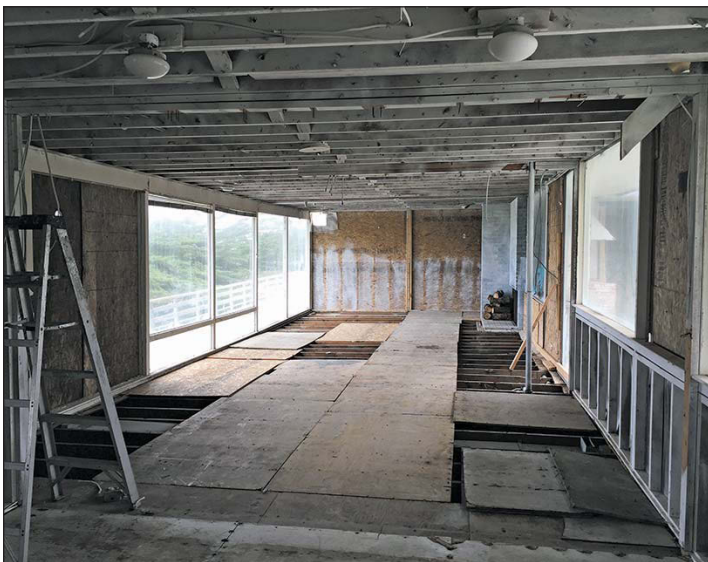
The dilapidated historic Pebble Beach house owned by Massy Mehdipour has been gutted by order of the county to make it possible to protect its structural elements. Mildew-resistant paint has been applied to the interior, including the living and dining rooms, as shown here.
