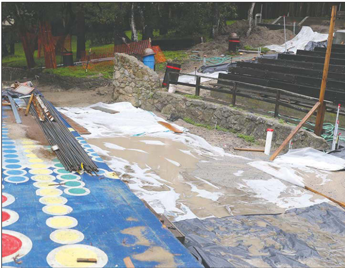
Substantial winter rains caused some delays in the renovation of the Forest Theater, which was originally set to be completed last November but is now anticipated to be done by the end of March.
