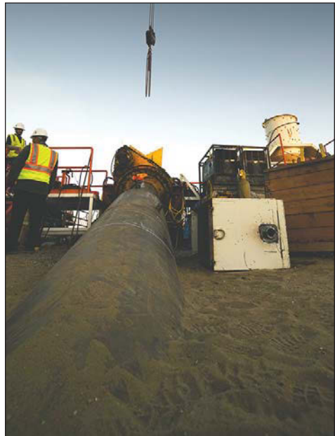
A desal test well being drilled in Marina. Candidates for county supervisor disagree about how big a new desal plant might have to be.
