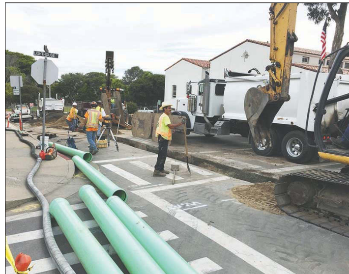
Tuesday in P.G. yet another major artery through downtown was closed for sewer replacement — this one alongside the post office. It's a scene that's happened on many streets over the last few weeks, but is almost a thing of the past, according to a city official.
