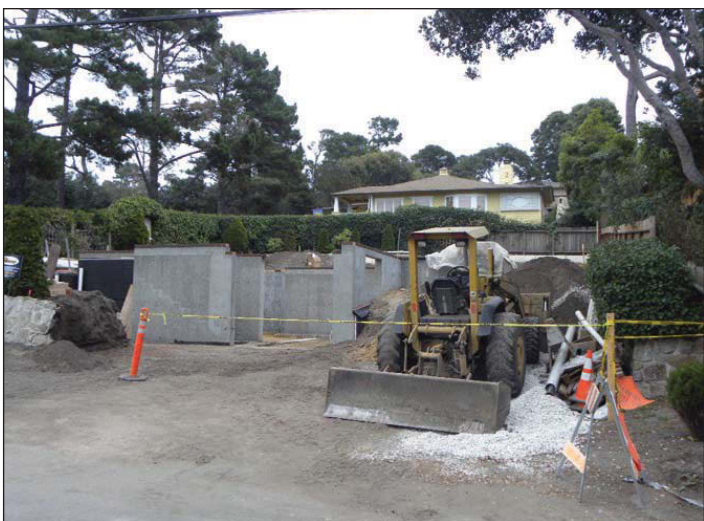
A cistern at the home of Bill and Adriana Hayway on Carmelo Street was approved by the planning commission earlier this month, even though it will be in the setback, which is normally off-limits to structures.
