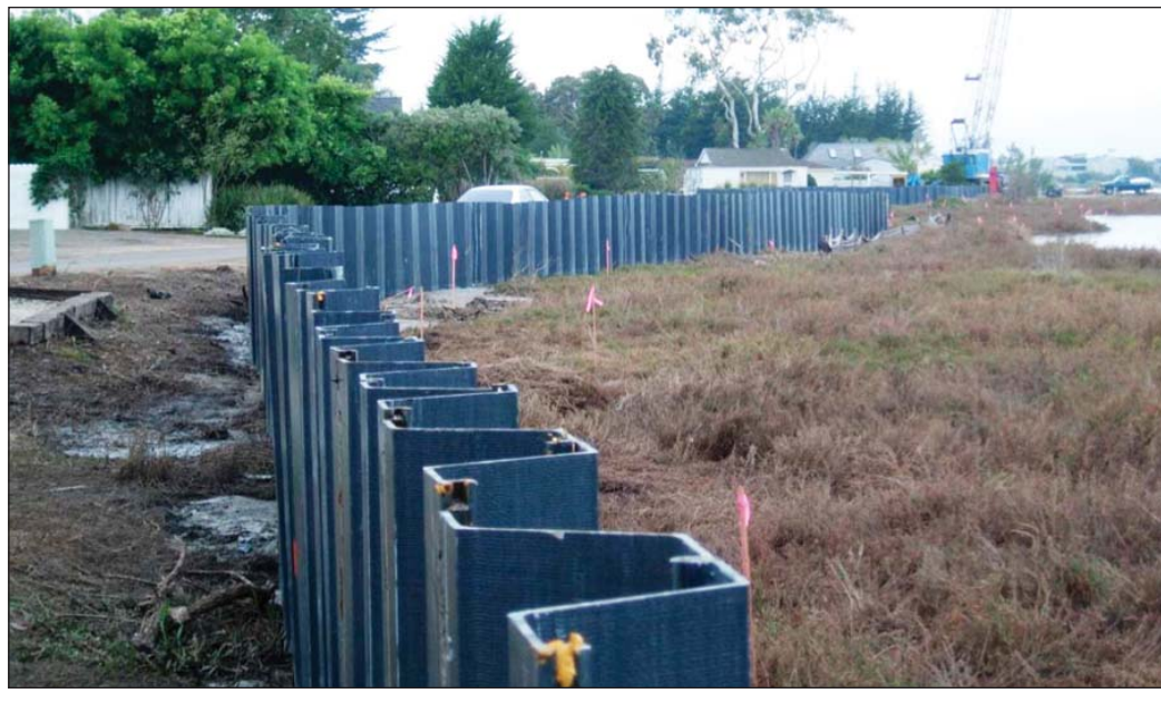
A sheet-pile lagoon barrier in Carpenteria similar to the one proposed for the north side of the Carmel River Lagoon.
