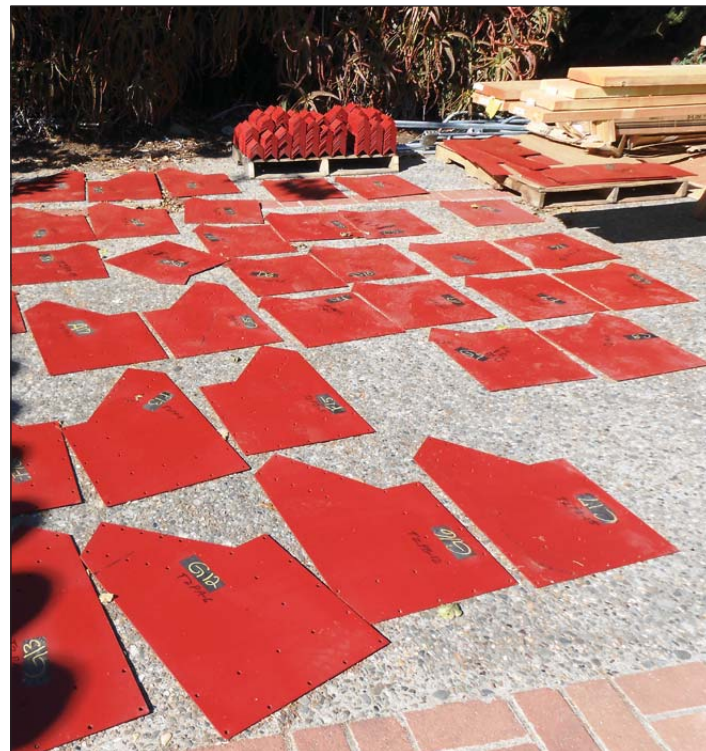
High-tech 3-D imaging allowed contractors to precisely cut these steel plates, which are being used to strengthen roof members on the Mission Basilica.
