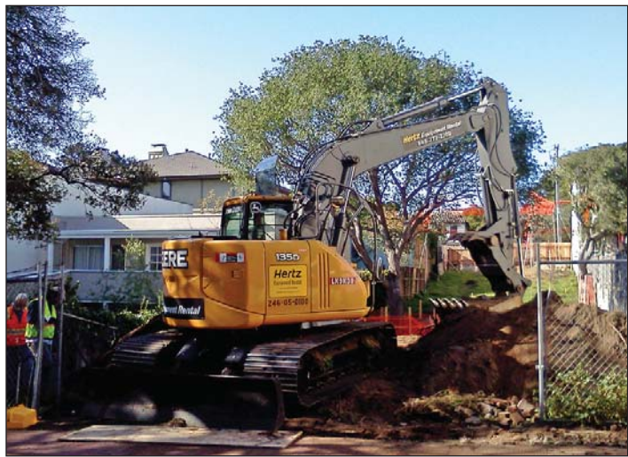
Excavation has begun for the first of two duplexes being built by property owner Don Mackey downtown.
