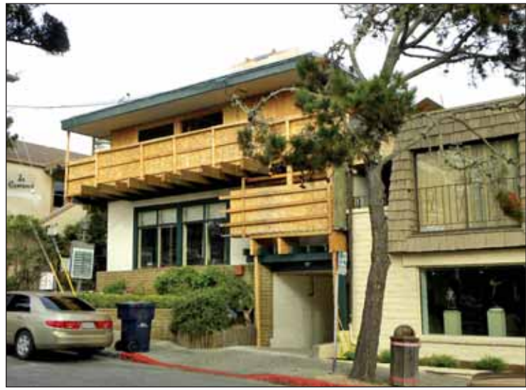
Construction is under way on the new upstairs apartment in Su Vecino Court. Due to its flat roof and contemporary design, the owner will be allowed to install aluminum-clad windows in it.
