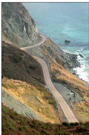
Pitkins Curve is one of the worst sections of Highway 1 Big Sur for rock slides.
