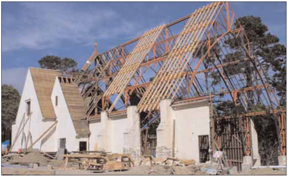
The $21.65 million reconstruction of Sunset Center was a really big deal and included demolishing much of the former school auditorium and rebuilding it from scratch while retaining important historic elements. Shown here is the new auditorium being framed in early 2002.
