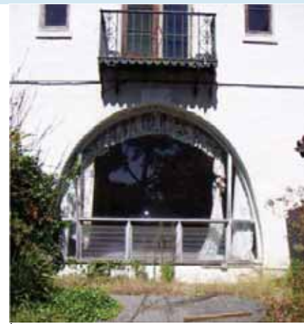
Current State of Decay
