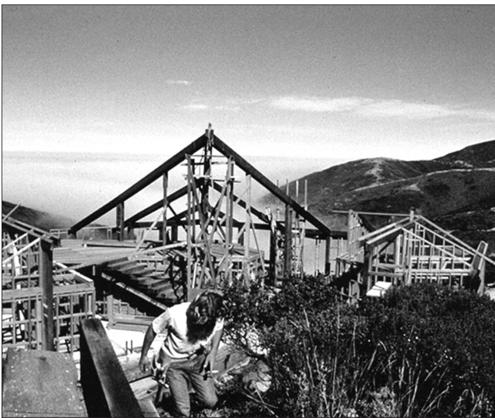
During construction, fog often rolled in over Pfeiffer Beach far below, but the house being built on the ridge was high enough to remain in the sunshine.
