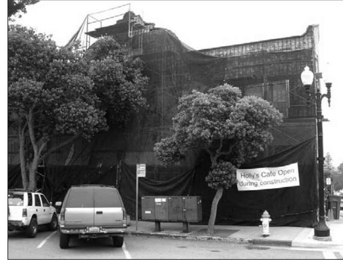
Construction crews found old tin siding and iron columns while remodeling this commercial building at 601 Lighthouse Ave. in Pacific Grove.
