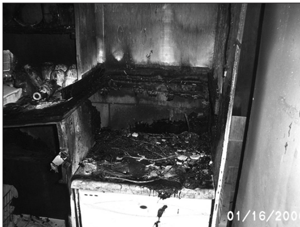
The charred area above a dishwasher in a hotel laundry room shows the origin of Monday's fire.
